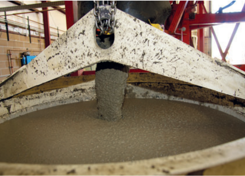
Fig. 6: Consistent SCC mix flows from the ACT HPGM mixer into a crane bucket at the Trenwa Colorado precast plant. Operators can call for or adjust batches from a remote call panel located near the mixer platform. High flowability of SCC has allowed Trenwa to eliminate vibration and is helping to reduce the average shift from 10 hours to 8.
