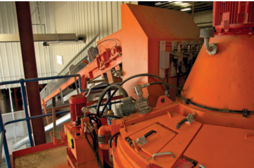
Fig. 2: Wiggert HPGM 1125 mixer with aggregate batch transfer conveyor (at left) charges the mixer. The HPGM 1125 mixer is equipped with an automatic high pressure mixer cleaning system. This system saves Trenwa about 30 minutes per shift in clean out time and ensures good housekeeping for longer mixer life.
